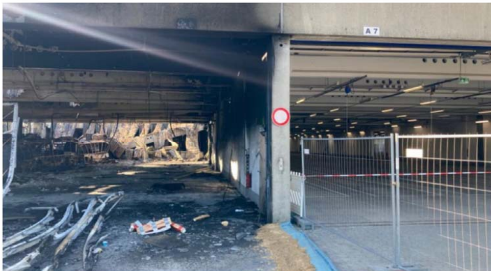
Figure 2: Fire in a depot hall divided by fire walls: Fire section on the left affected by the fire, adjacent fire section on the right without the effects of the fire. Buses from this area remained unharmed. (Image source: ÜSTRA, Hanover)
