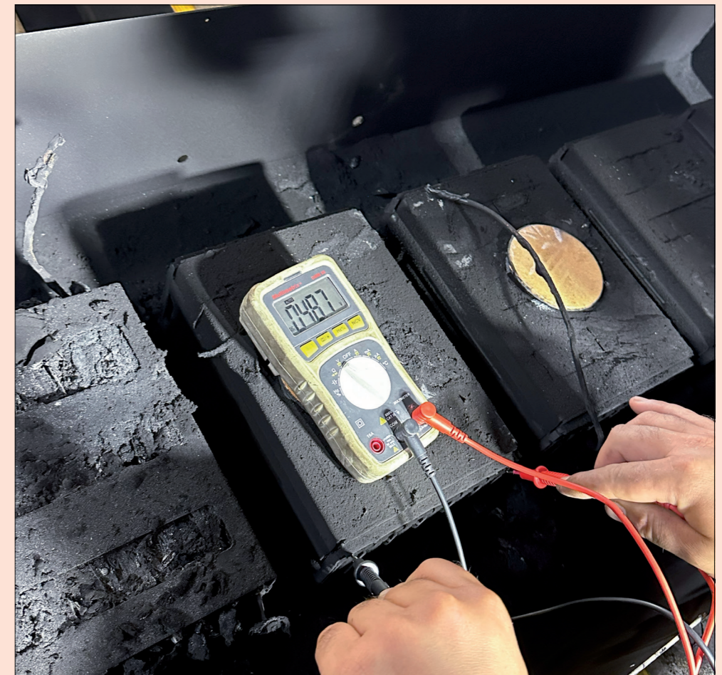
2024: Testing on simulated BESS: Battery module voltage – 3 hours after
