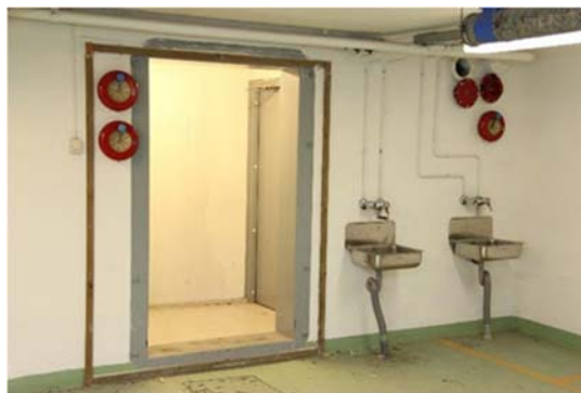
Figure 15: Water points are visible next to the entrance to the civil defense shelter, as well as ribbing around it for the construction of a lock tent. The lock tent serves as a vestibule for the shelter.
