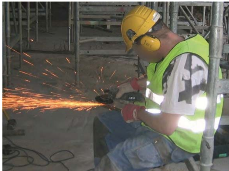
Figure 5: Risks related to repair and modification work can be reduced with sufficient planning. Special attention should be paid to hot work safety.
