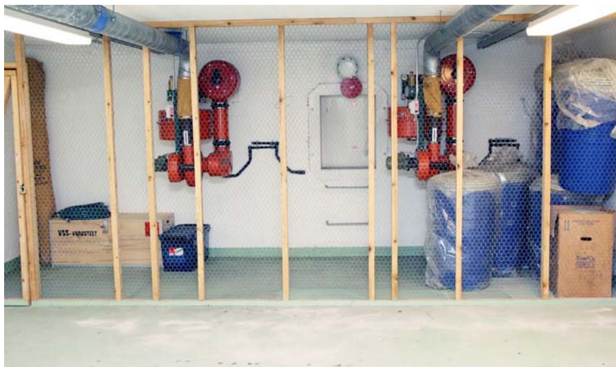
Figure 1: A civil defense shelter. Civil defense shelters are more common in Nordic countries. It is recommended to appoint a shelter manager and their assistant for each civil defense shelter.
