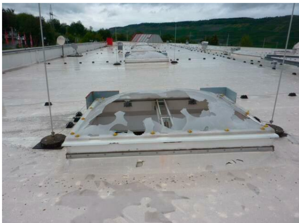
Figure 4 Example of a skylight and plastic roof foil cover destroyed by hail (source: GDV)
