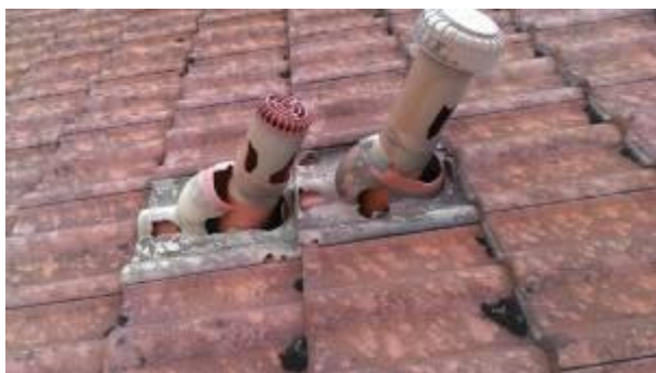
Figure 8 Roofing exhauster as additional roofing equipment damaged by hail (source: EPZ)
