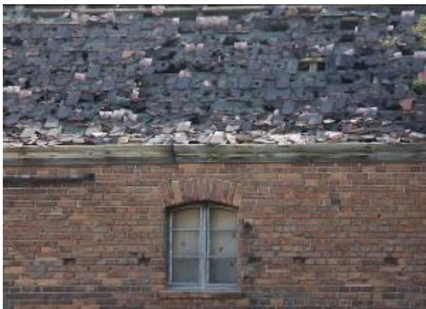
Figure 3 Example of roof destroyed by hail (source: GDV = German Insurance Association)
