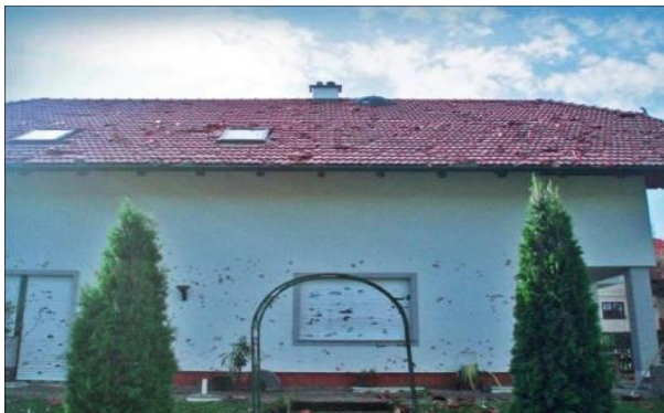
Figure 2 Example of damages on building (source: EPZ)
