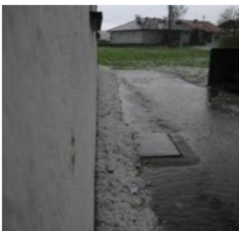
Figure 13 Many small hailstones block dewatering systems (source: EPZ)
