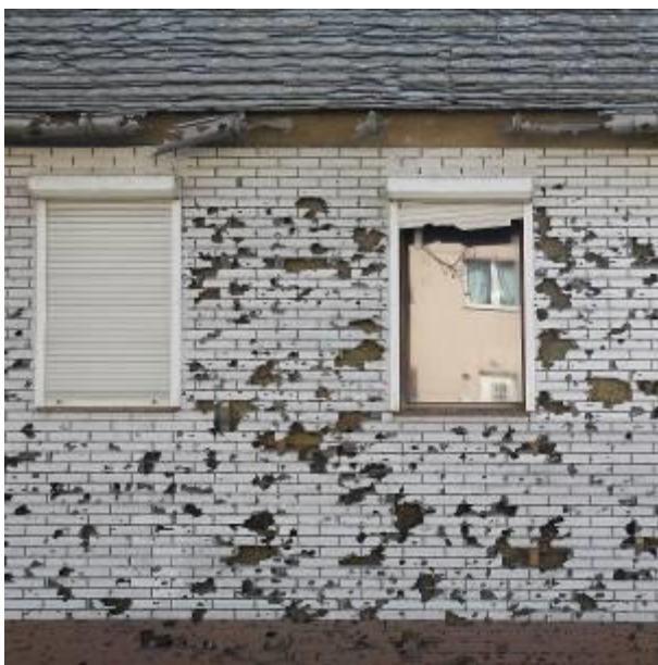
Figure 12 View of a facade destroyed by hail (source: GDV)
