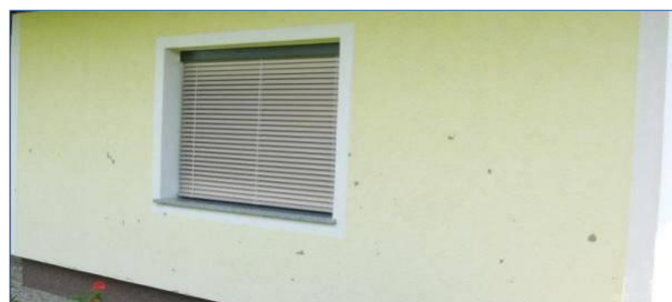
Figure 10 Thermal insulation system damaged by hail (source: EPZ)
