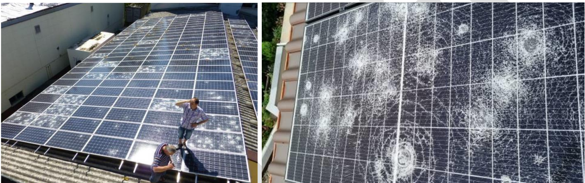
Figure 5 Example of some PV models partly damaged by hail (source: GDV/EPZ)
