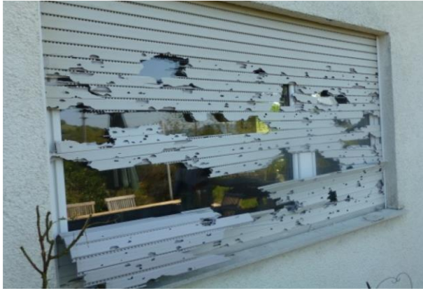
Figure 11 Plastic roller shutter for windows destroyed by hail (source: GDV)
