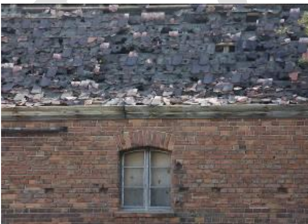
Figure 3 Example of roof destroyed by hail (source: GDV)
