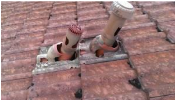
Figure 8 Additional roofing equipment damaged by hail (source: EPZ)
