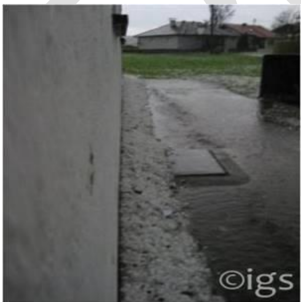
Figure 13 Many small hailstones block dewatering systems (source: EPZ)
