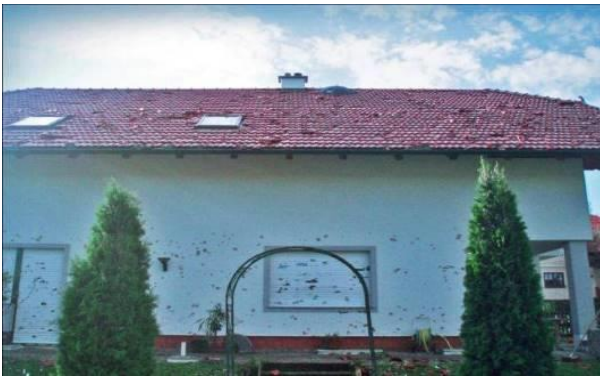
Figure 2 Example of damages on building (source: EPZ)
