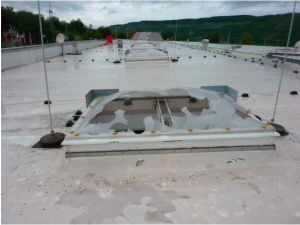
Figure 4 Example of a skylight and plastic roof foil cover destroyed by hail (source: GDV)
