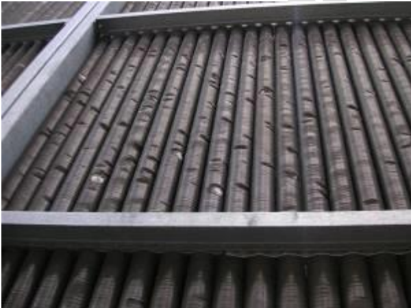
Figure 6 An air condenser system on roof damaged by hail (source: GDV)
