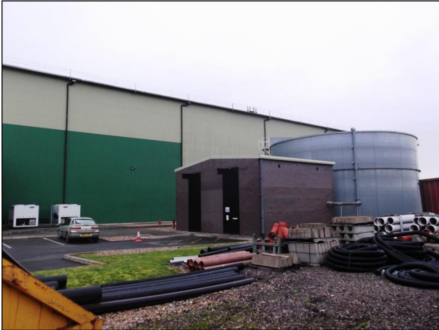
Figure 3: The best solution – a dedicated water storage tank.
