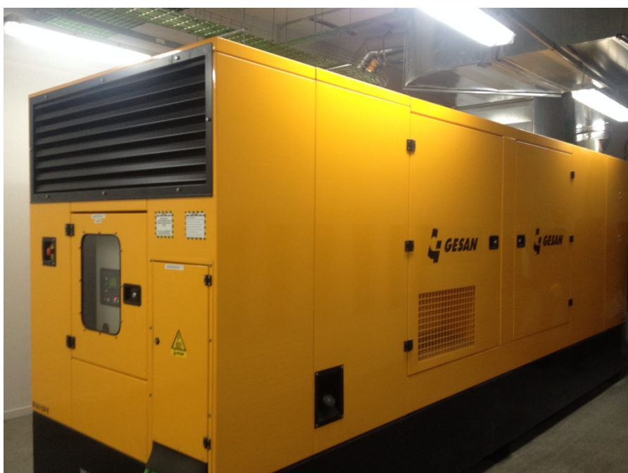
Photo1: Fixed generator installed within a building.
