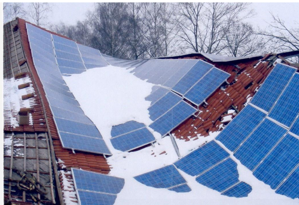
Figure 1 A montage of photovoltaic panels on the roof together with a lot of heavy snow can easily overload a roof above its design parameters and result in collapse. Photo: GVD, Germany
