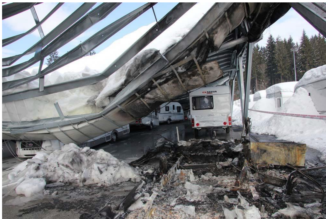
Figure 2 Damage because of heavy snow load can result in very high cost. Photo: Breda Dušič Gornik/Dolenjski list
